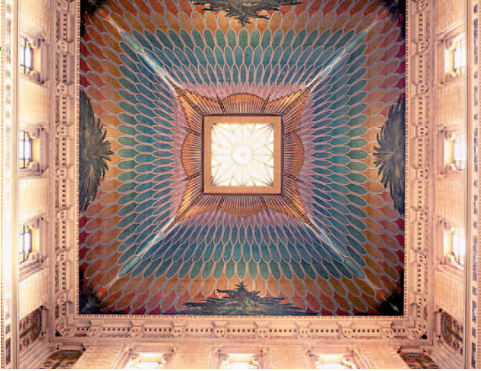
The ceiling of the neo-Babylonian Synagogue of Rome is decorated with ornate metalwork and frescoed palm trees.
